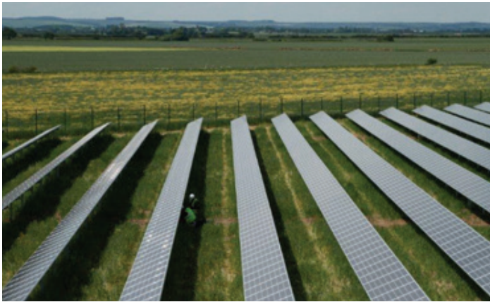
Figure 6 Adequate spacing between rows of panels is necessary to avoid overshadowing. Vegetation will grow between these rows and this vegetation will require management.
