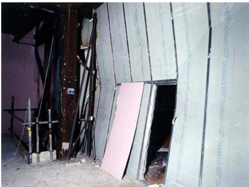
Figure A10 Stability failure of compartment wall (unexposed face) – BRE large compartment test
