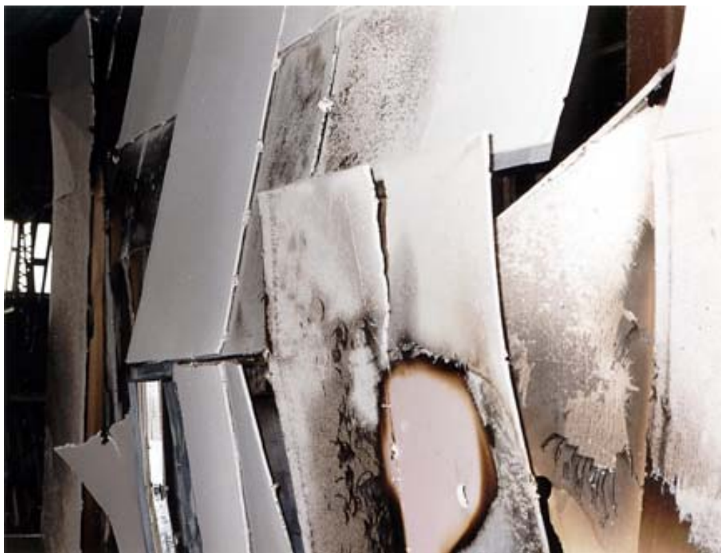
Figure A11 Integrity failure of compartment wall – BRE large compartment test
