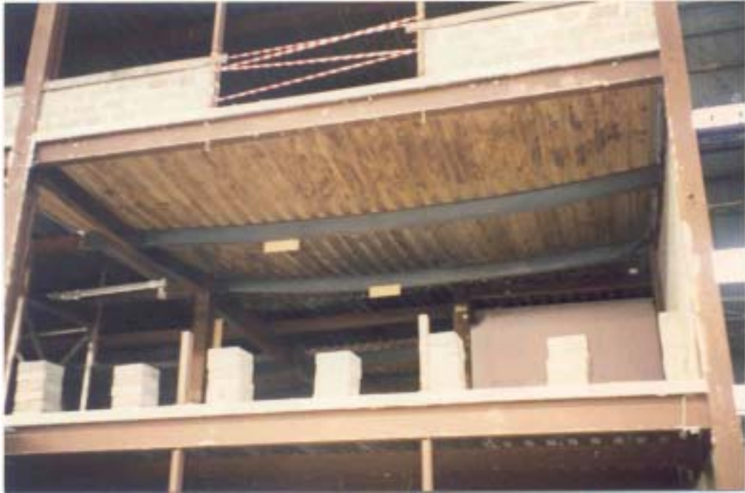
Figure B15 British Steel corner fire test – damage to steelwork and displacement of floor slab
