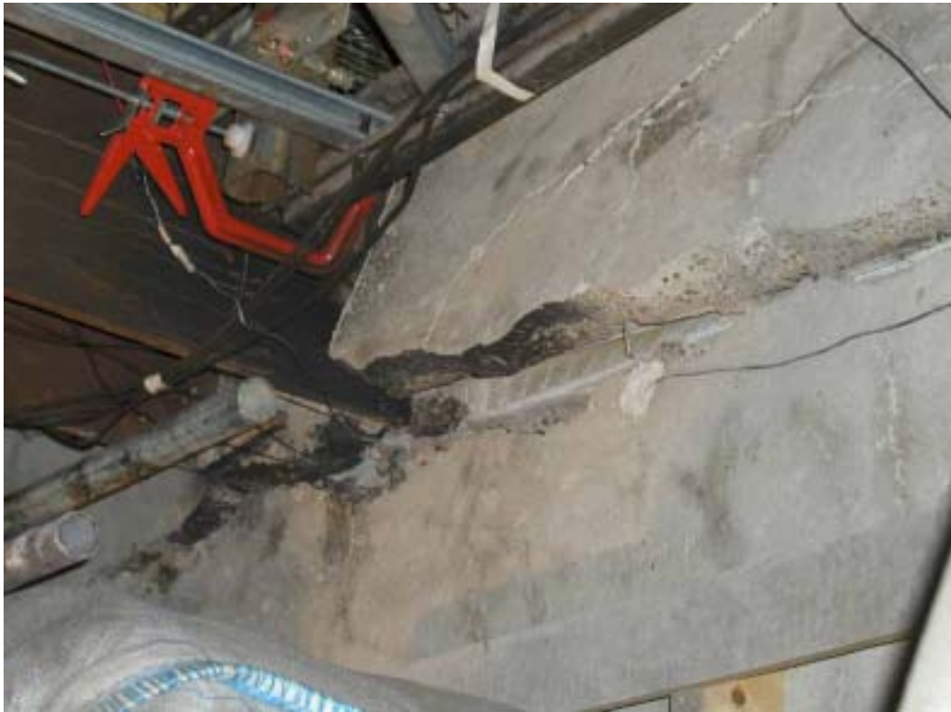
Figure B26 Cracking around internal column – European connection fire test
