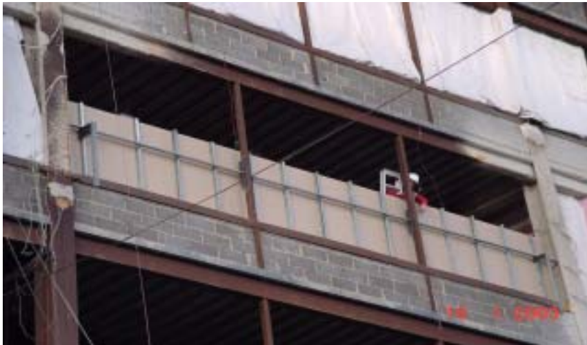
Figure D3 Fireline plasterboard over window opening
