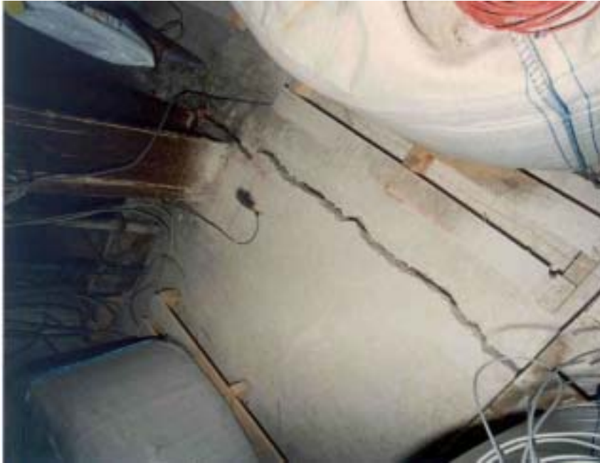
Figure B20 Cracking of floor slab – BRE large compartment test
