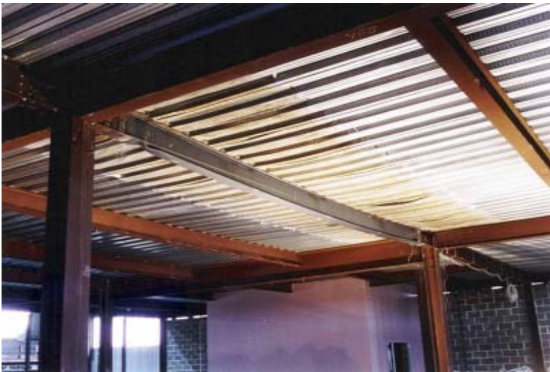
Figure B4 Restrained beam post-test
