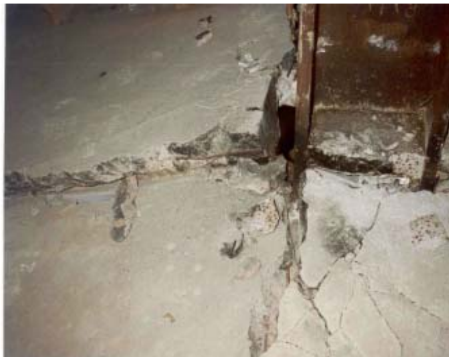
Figure B21 Integrity crack around column – BRE large compartment fire test
