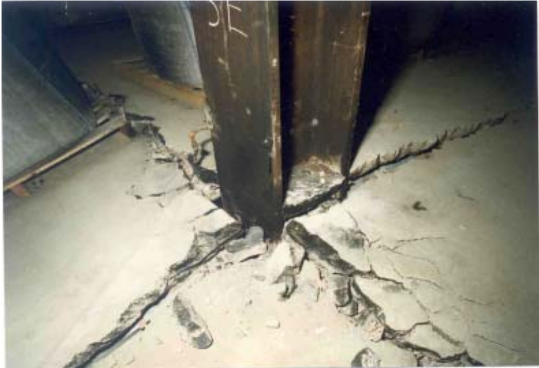
Figure B23 Cracking around column E3 – British Steel Demonstration Test
