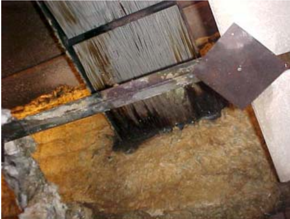
Photograph B13. Fire spread from the underside of the cavity barrier.
