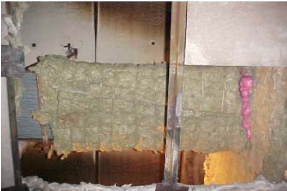
Photograph B8. Fire stopping adjacent to the cavity barrier also shows the wrapping around the cables.
