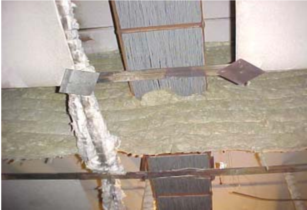
Photograph B3. Cable ladder running through the cavity barrier.
