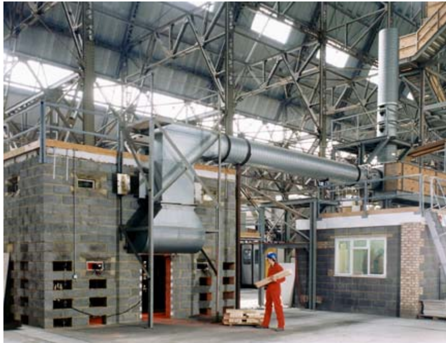
Photograph B1. BRE Real Scale Cable Fire Test Facility
