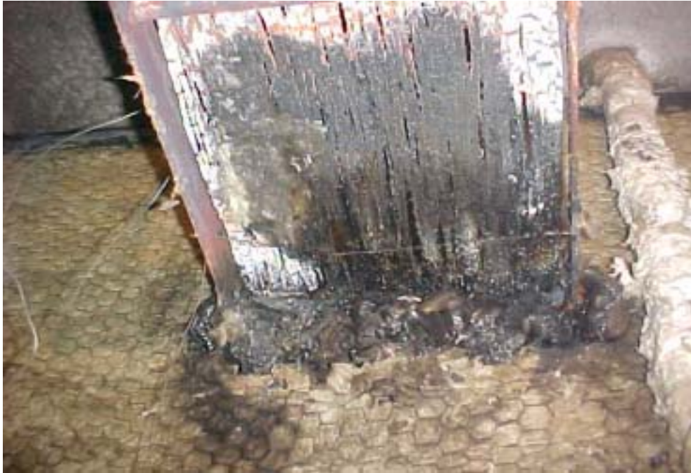
Photograph B11. Underview of the cavity barrier with fire stopping around the cable ladder.
