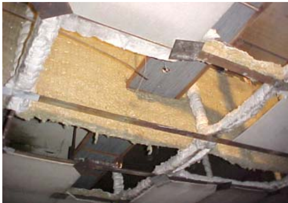
Photograph B4. Cable ladder running through the cavity barrier.
