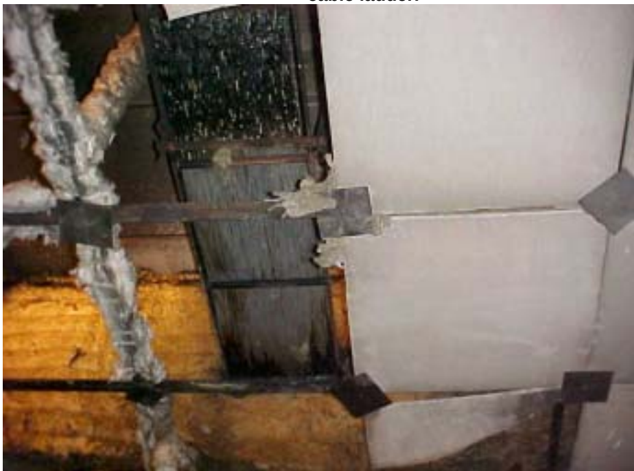
Photograph B12. Burner flame impingement on the cable ladder
