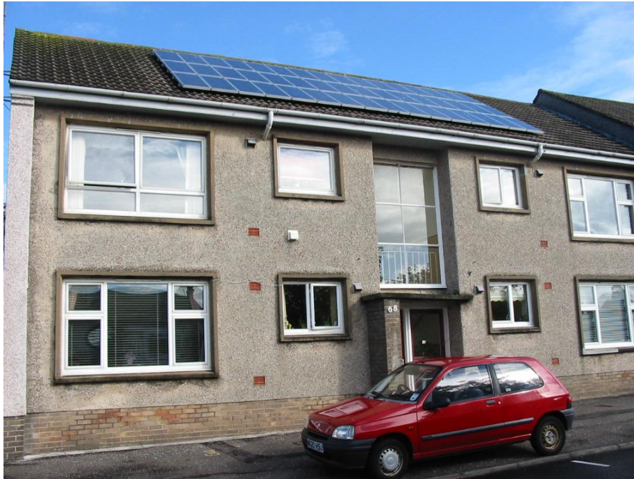
Figure 28: The PV array mounted on the pitch roof using the Intersol mounting system
