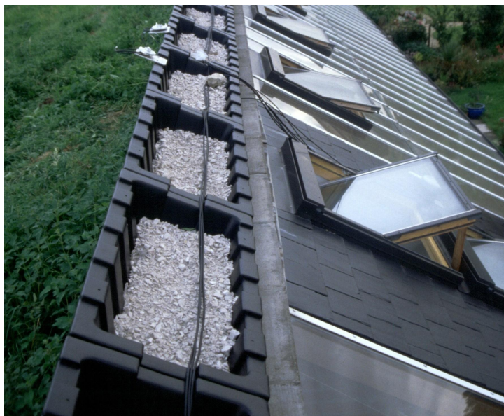
Figure 31: Ballast levelled off, dc cabling installed and irradiance sensors for monitoring equipment installed (Hockerton Housing Partnership)
