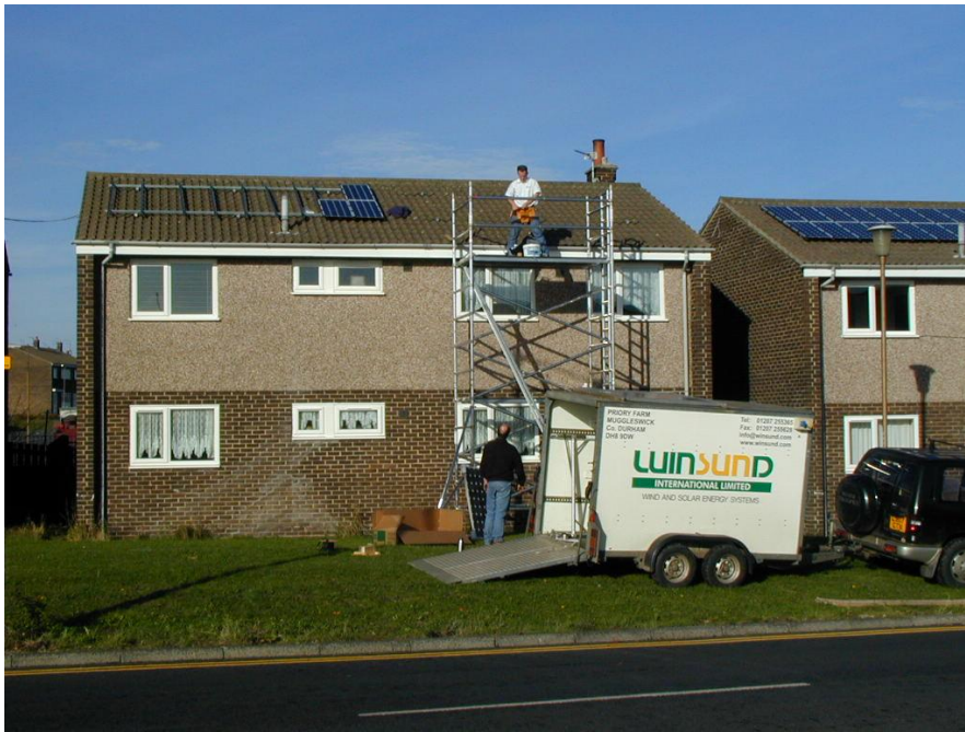
Figure 20: Using scaffold tower to install the “Sun-in-a-box” system: laminates portrait, base structural rails horizontal
