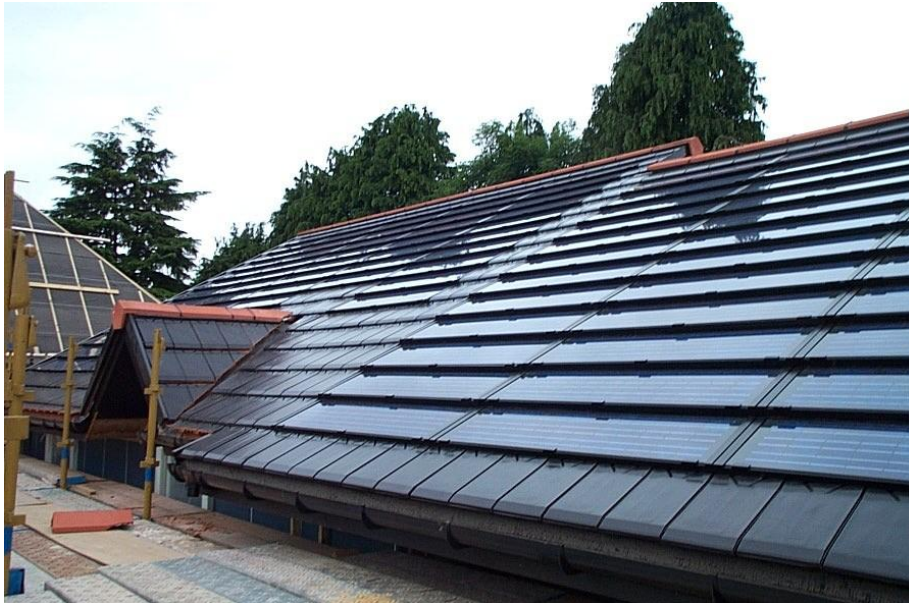
Figure 5: View of the Pfleiderer Terra-Piatta solar roof tiles on a number of adjoining properties
