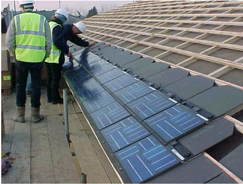
Figure 3: The third row is installed and the tiles connected up by the roofer (photo – Laing Homes)
