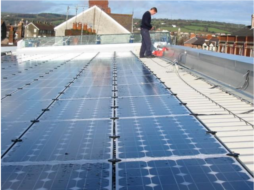
Figure 30: View of the installed modules on the roof top
