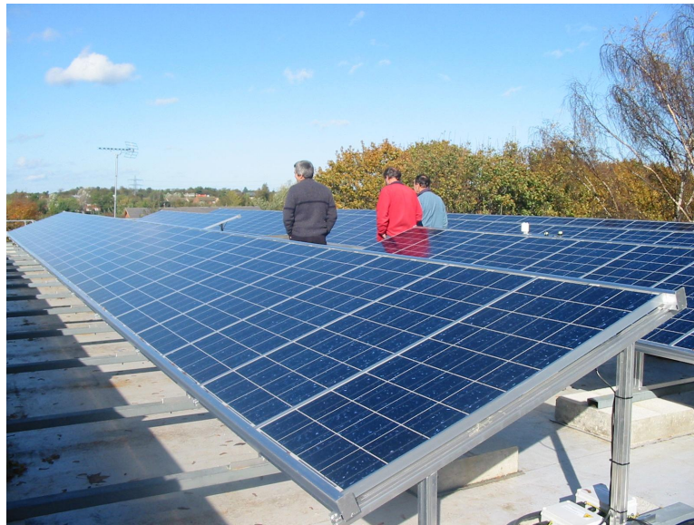
Figure 32: The installed frame-mounted PV system
