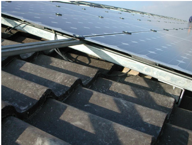
Figure 22: Looking along the PV array as it is being installed, showing the steel channel and the “diamond” fixings
