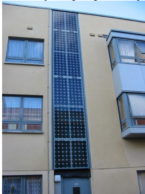
Figure 33: Façade Integrate System in place using some “dummy” PV panels where there is increased shading
