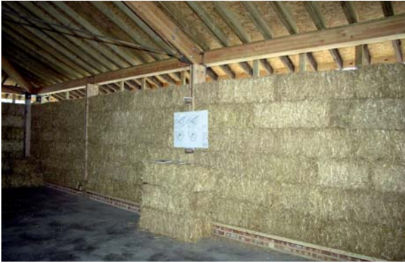
Figure 6: Six courses of straw bales laid in stretcher bond with the seventh about to be added (Courtesy of Mike Beckett/Collins & Beckett)
