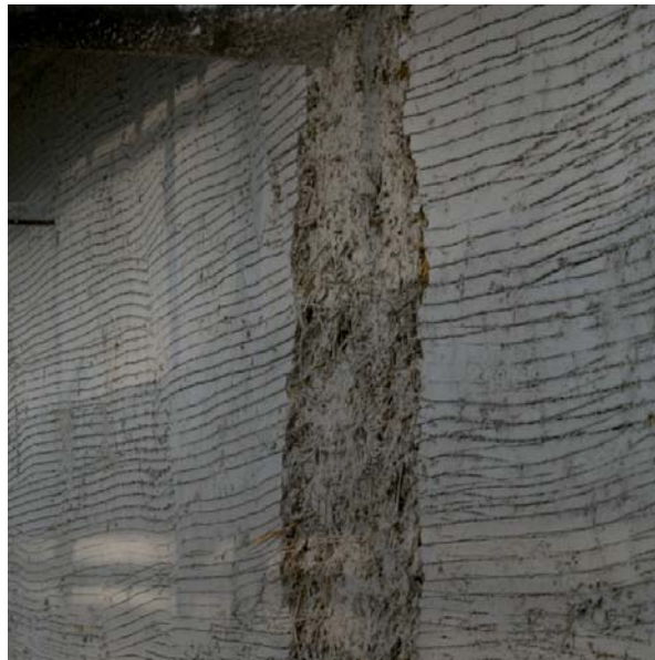
Figure 10: Second coat of render has been applied (Courtesy of Mike Beckett/Collins & Beckett)
